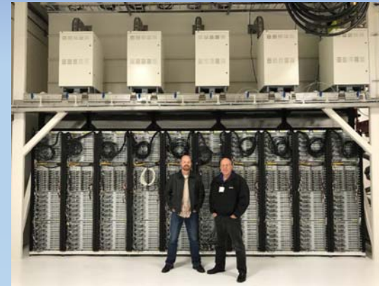
Fuel cells in Microsoft “datacenter of the future”
